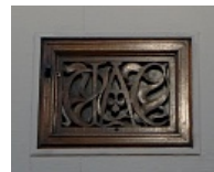
Fretwork cover of ventilation duct incorporation the letters G, A and C.
